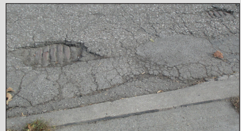
Existing potholes exposing original brick street
