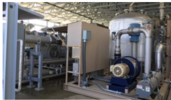
Landfill gas collection at the Bluff Road landfill.
