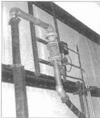
Residual water metering
