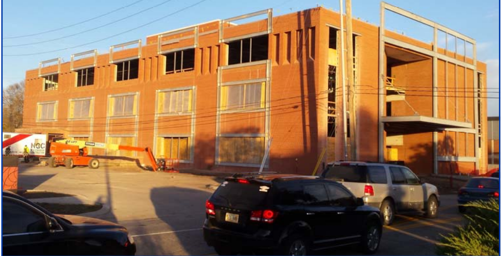
Construction is well underway on the 401 Building, the first phase of the Telegraph District , on the southwest corner of 21st & L Street. Formerly windowless, the building is being completely rehabbed inside and out. Nelnet will move into the 401 Building in early 2017 and eventually employ up to 700 employees at that location.
