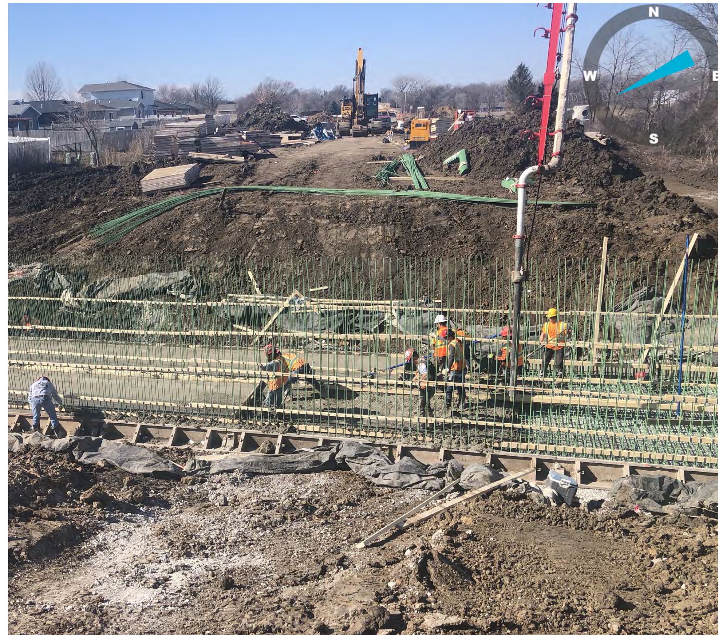
Box Culvert Between SW 30th & SW 27th - Rebar, Forming Sides, Placement & Pouring Box Floor
