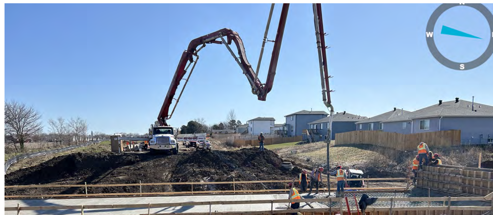
Box Culvert Between SW 30th & SW 27th Deck Being Poured, Formed & Poured Walls
