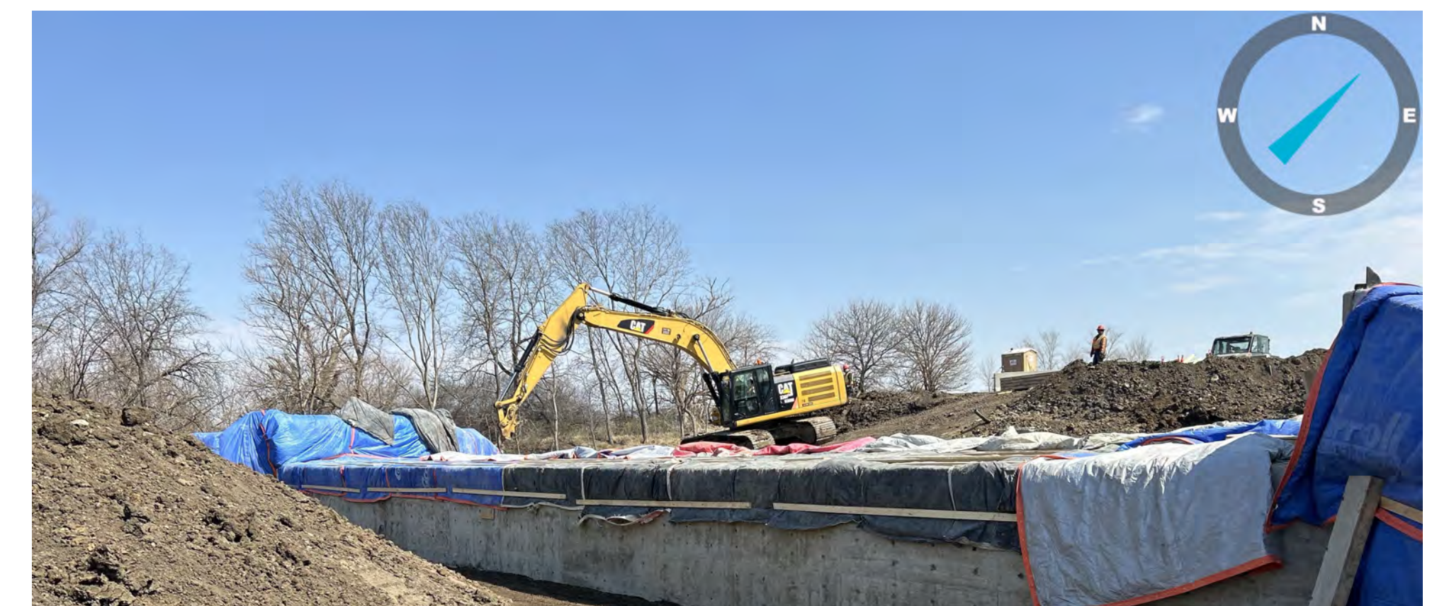
Box Culvert Complete Between SW 30th & SW 27th - Curing Stages & Dirt Work & Backfilling Operations
