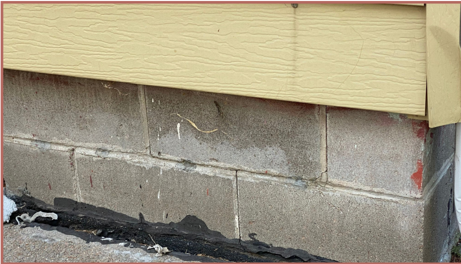
Smooth concrete block foundation which departs from the original look of the rock-faced concrete block.
