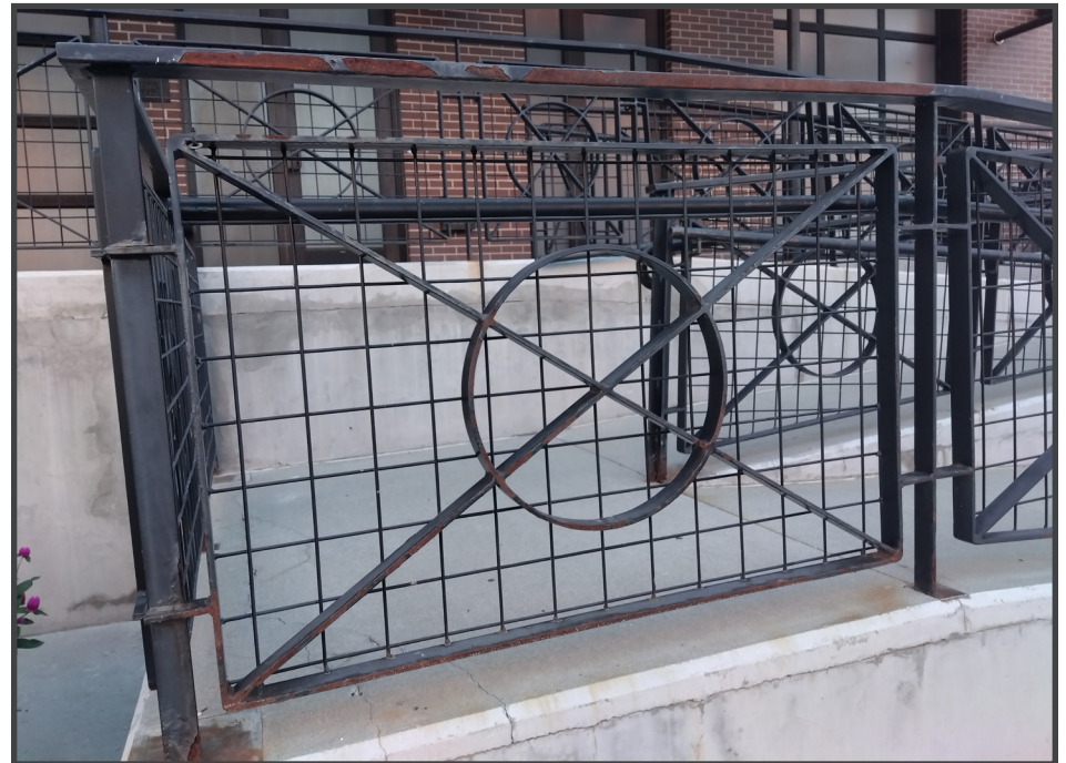
Dock railing example commonly found in the Haymarket Historic District with a simplified design. Given the rust showing, the metal type used on future projects should be looked at for compliance with the guidelines.
