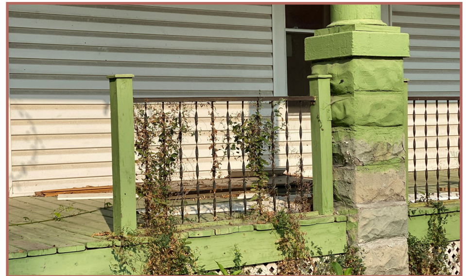
These railings are not compliant with the guidelines, with a modern metal spindle going directly to the porch floor. The stone column base should also not be painted.
