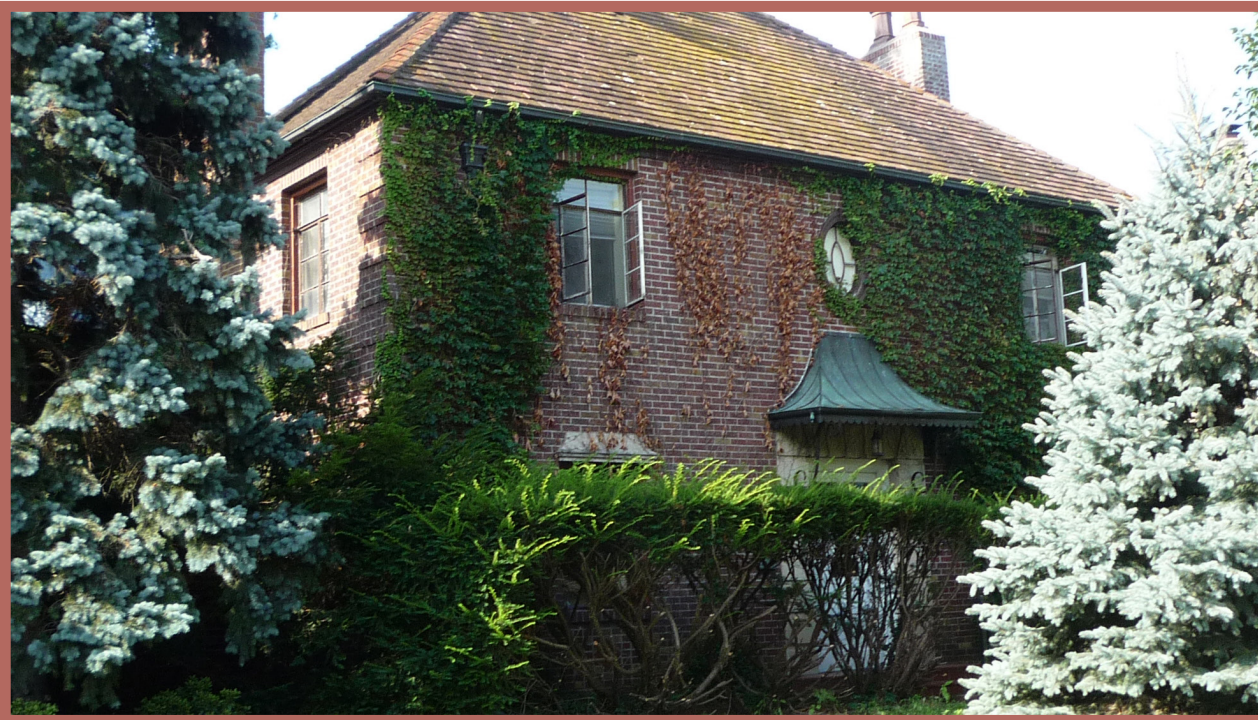
The landscaping has grown to a height that obscures first floor windows and the vines are growing over second floor features.
