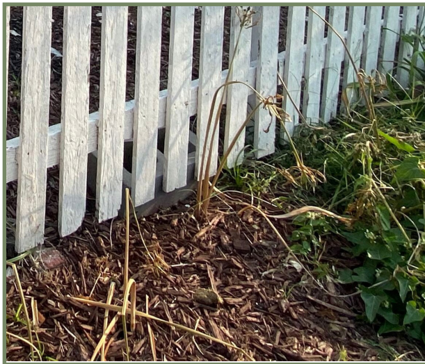
Example of a fence less than 48 inches in height with greater than 50 percent opacity.
