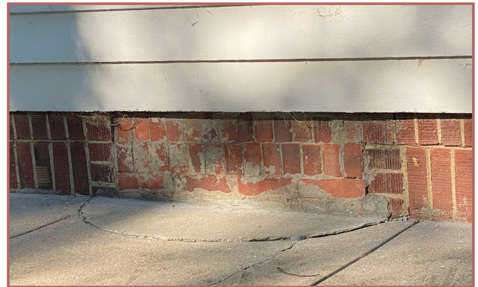
Improper blocking in of basement window
