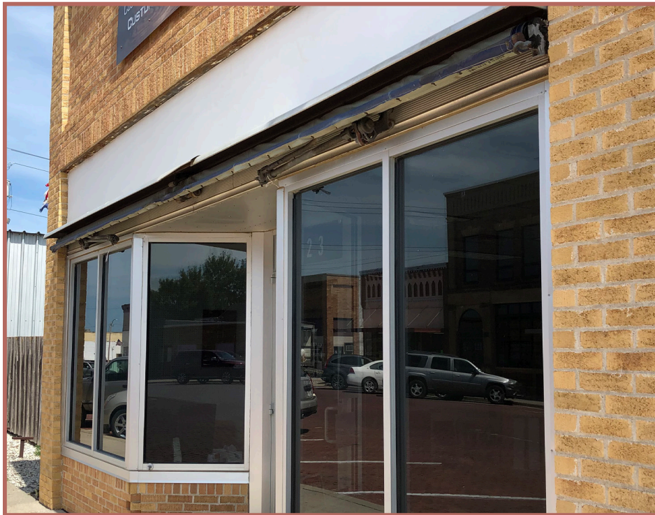
The above storefront has a modern aluminum frame with the original roller awning intact above. The unpainted metal stands out from the buff brick facade and is not a recommended replacement.
