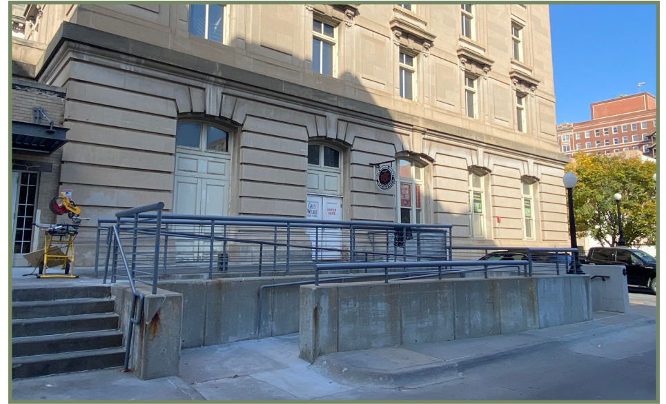
The image above shows the Old Federal Building with a ramp added to the rear of the building. The grey color of the railing does not compete with the building, however the amount of rails starts to interfere with the facade. It's location on the rear is ideal for a treatment of this level.
