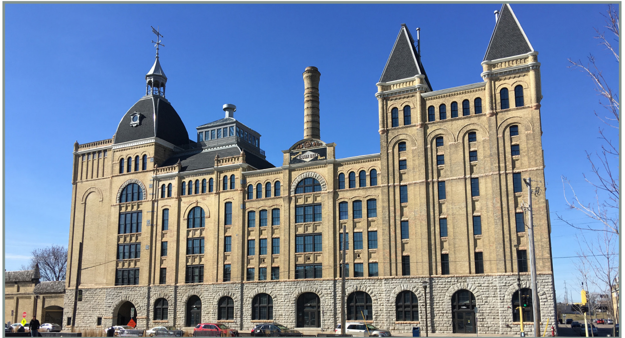
The synthetic slate roof on the Grainbelt Brewery in Minneapolis is nearly identical to the original slate roof given the height and scale of the building.
