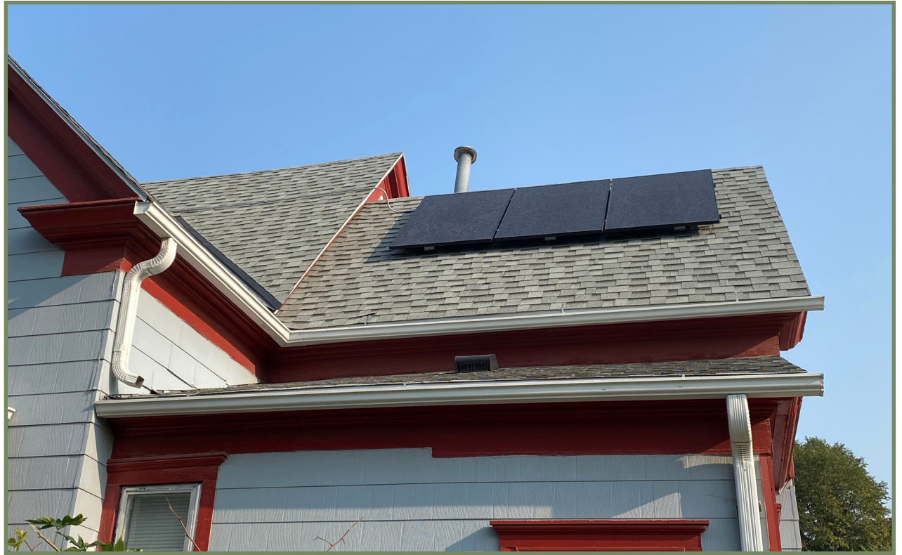
Solar panels mounted with a low-profile, flush against the slope, on a secondary slope.
